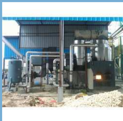
Solid Fuel Fired Hot Water Generator
