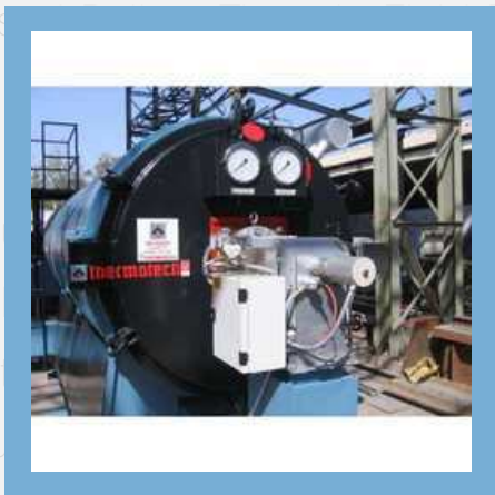
Thermic Heater-Gas Oil/Fired Burner
