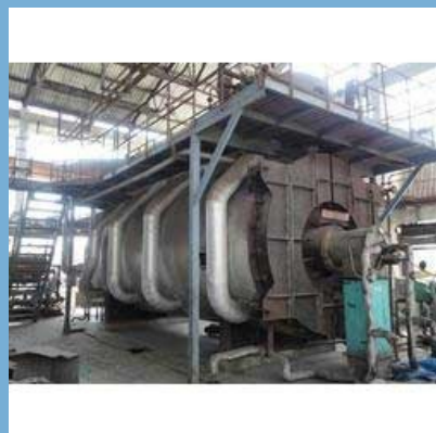
Oil Fired Boiler
