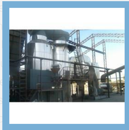
Thermic Fluid Heater - Solid Fuel Types of Grates
