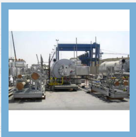
Hazardous Zone Thermic Heater
